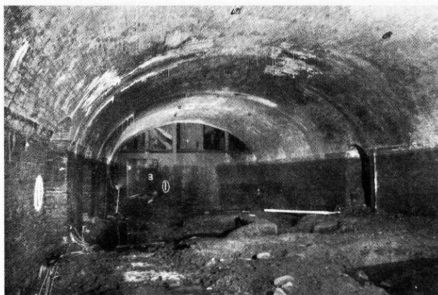
Plate 2 Engine room vault (BWCP)
